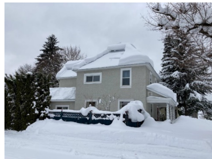
(H) Sliding snow causing unbalanced loading and accumulation on a low roof
