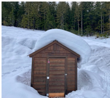
(G) Corncicing and unbalanced loading on a small shed roof
