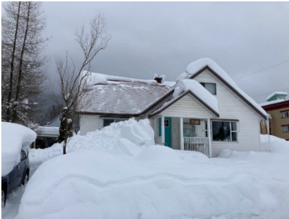
(C) Sliding snow causing unbalanced loading
